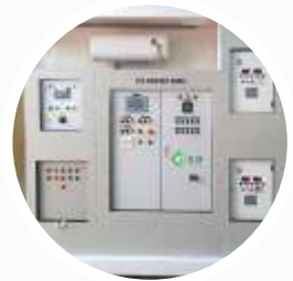
MCC & PLC Panel
